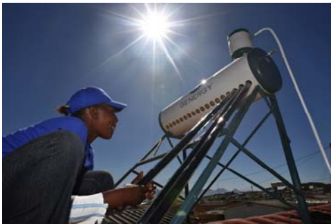
The solar water geyser - (Photo credit: Michael Goldman)
