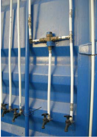
Tempering valve - (Photo credit: Michael Goldman)
